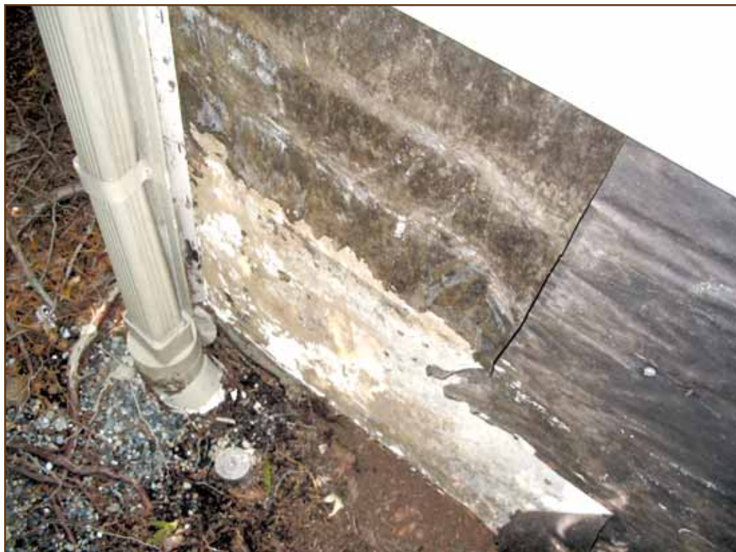
Photo 3 - Damage of gypsum sheathing terminating at grade (earth)
