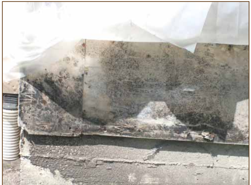
Photo 2 - Damage of gypsum sheathing due to water splash under siding
