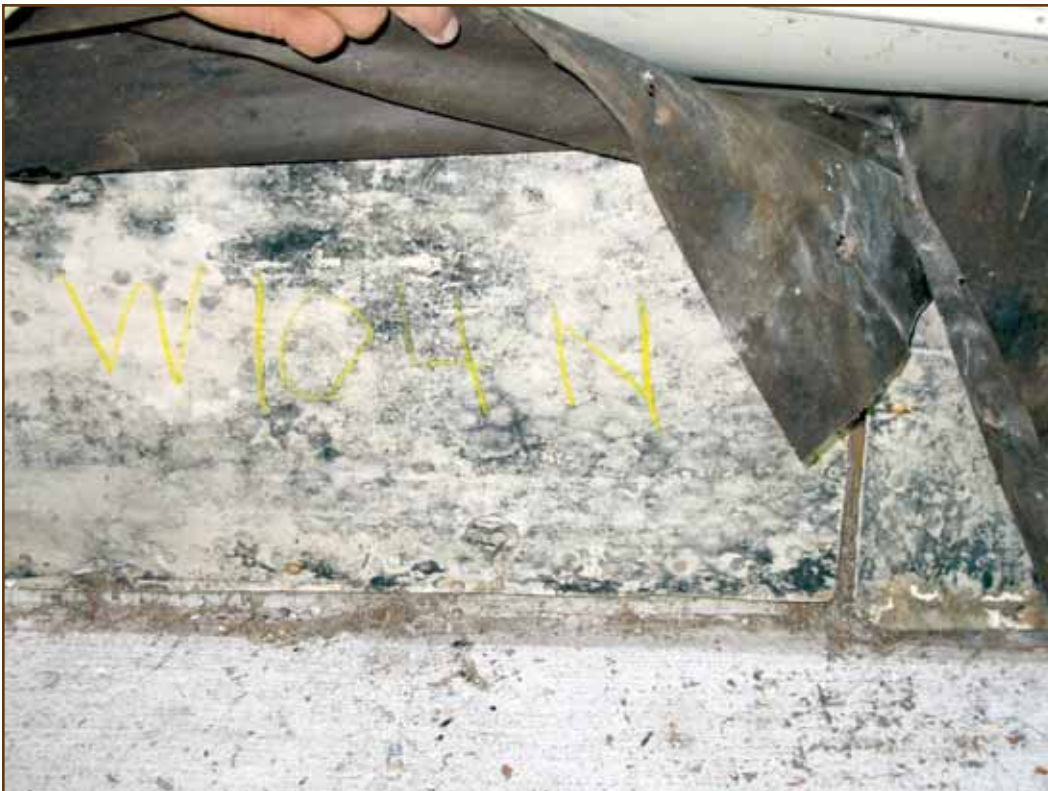
Photo 1 - Water and mold damage on gypsum sheathing terminating at hardscape
